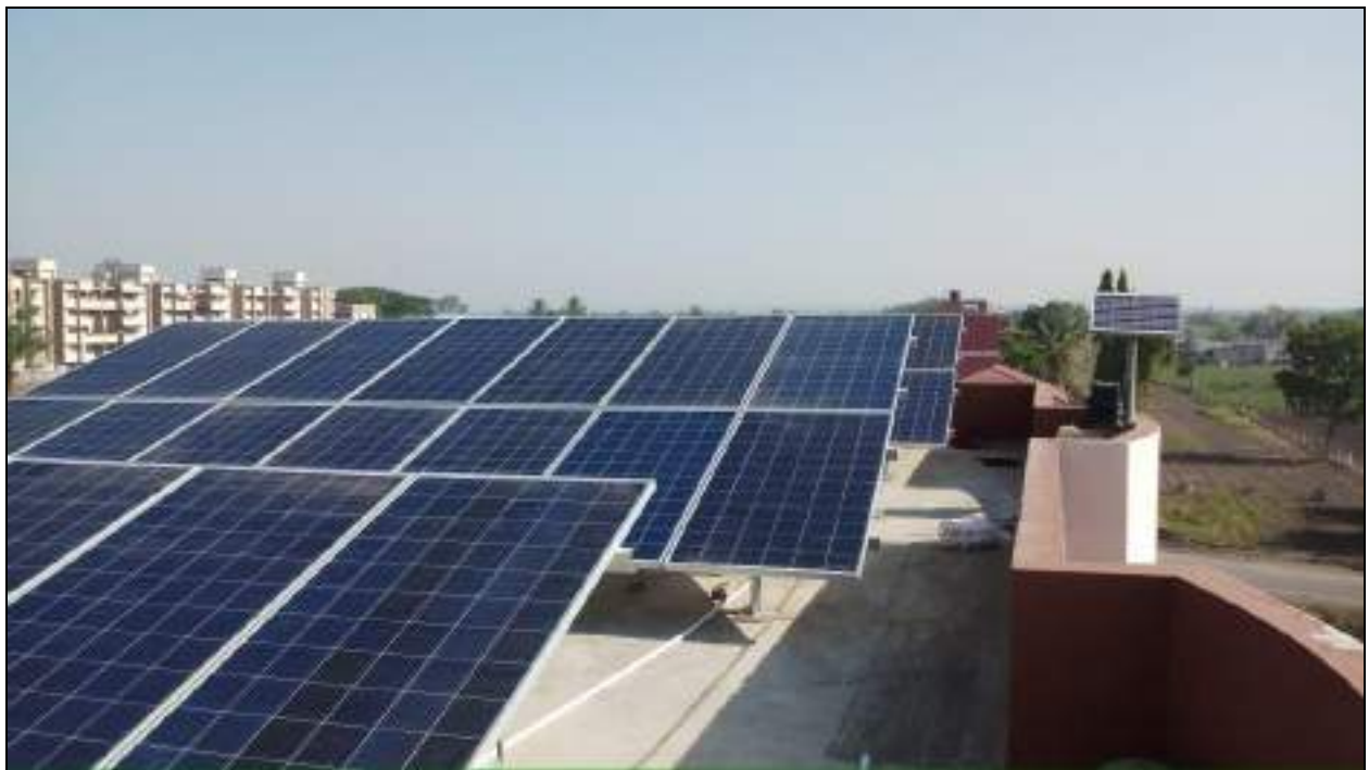
Micro-grid Installed at Maher Ashram: Vadhu Budruk Center
